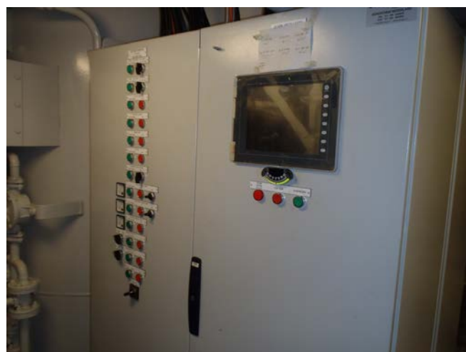
Main switch board
