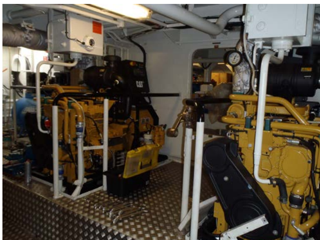
Generators PS and SB
