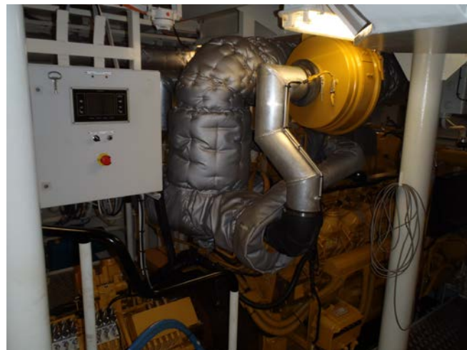
PS Main Engine towards gear box.
